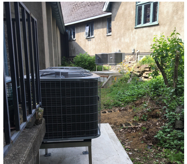
Outside portions of the air-source heat pumps used at Trinity Church, Ste-Agathe. A heat exchanger inside the basement furnace heats the church's forced-air system. Photo by John Richard.
