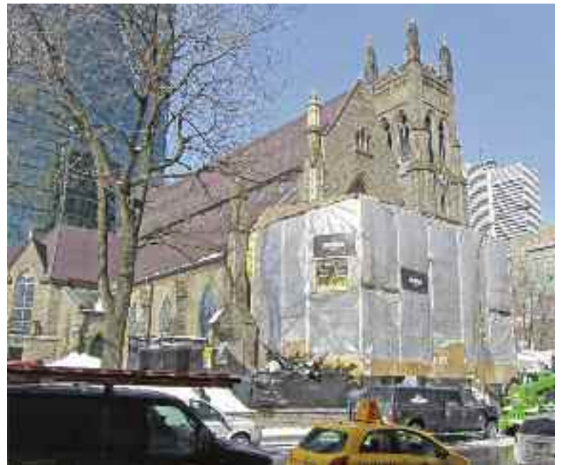
RENOVATION OF THE PORTICO of St. George's Place du Canada was well under way when federal subsidy was formally announced.
