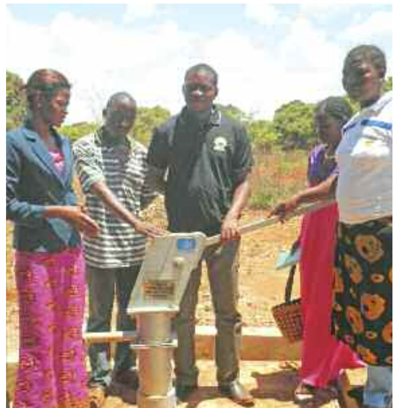
Several local Anglicans show off a new well pump installed by the Diocese of Masasi. It was funded by the Primate's World Relief and Development Fund and Canadian International Development Agency.
