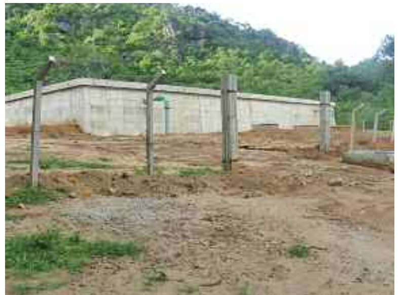
ONE OF THE CISTERNS. Behind it is the undisturbed foliage and in front all foliage has been removed. This cistern is only one of a series over a distance of about 25 kilometres between the well site and the town of Masasi. Just outside the picture on the right is the bishop's house.
