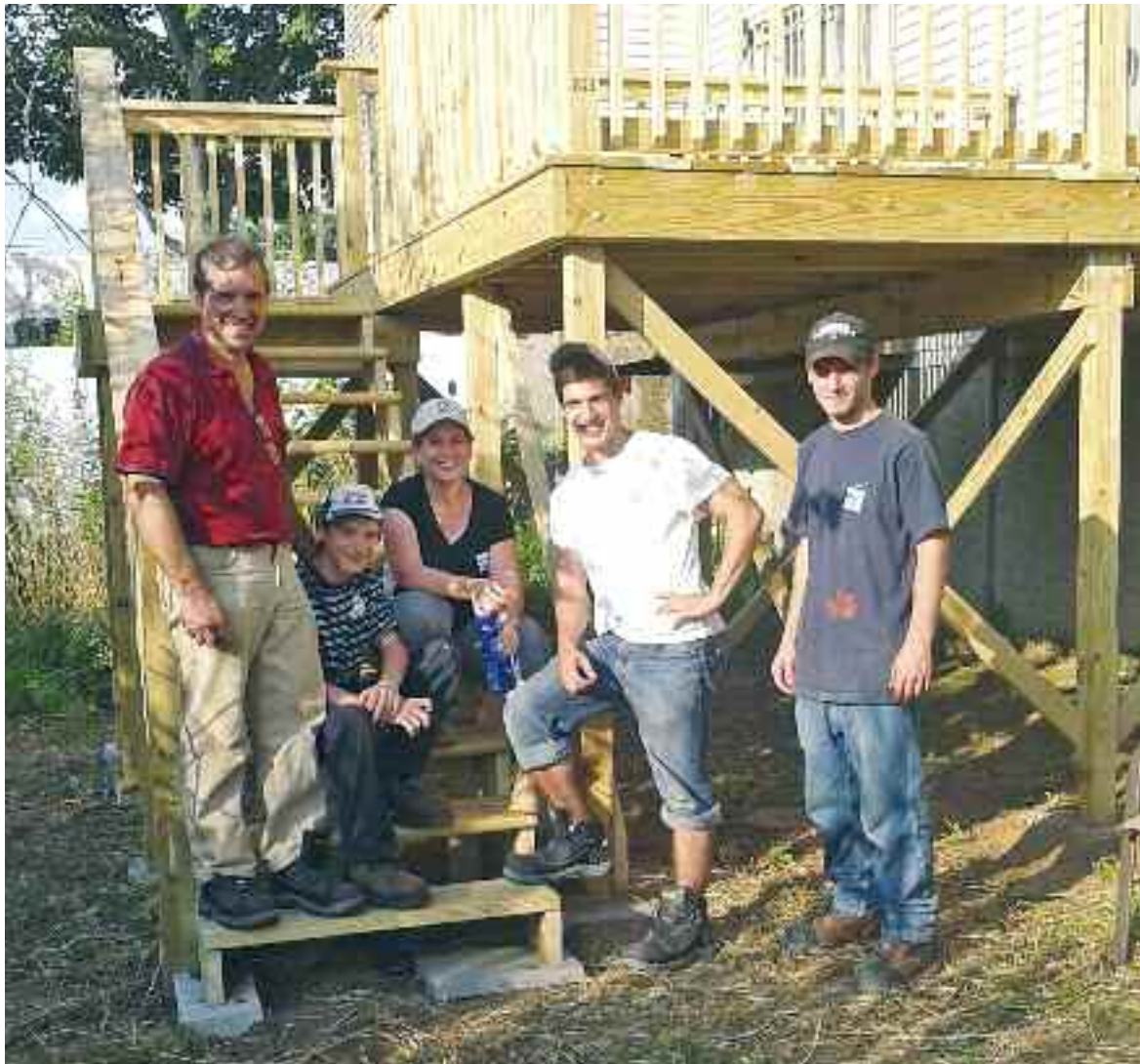
All decked out. The Amstutz family builds a new deck – to sea level. From left Andre, Ryan, Erin, Chris and Greg.
